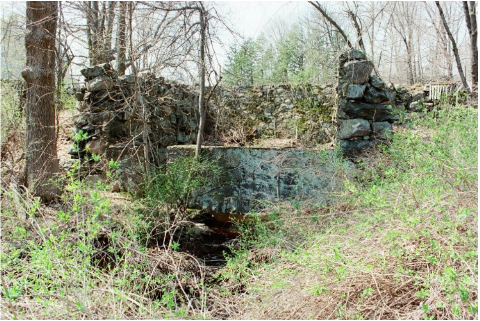
(Above) Mill site at 293 Boston Post Road, looking west (Photo by Cindy Bates)
