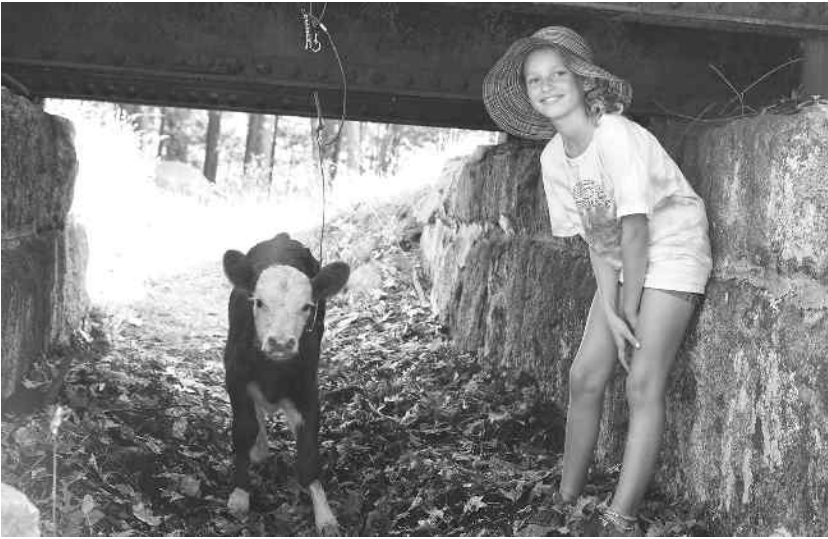
Demonstrating the function of the iron stringer cattle pass at Mile 14.81 is Chloe Sullivan, with a calf belonging to Alex Anza, a member of the Weston Agricultural Commission. (Photo by Gloria Cole)
