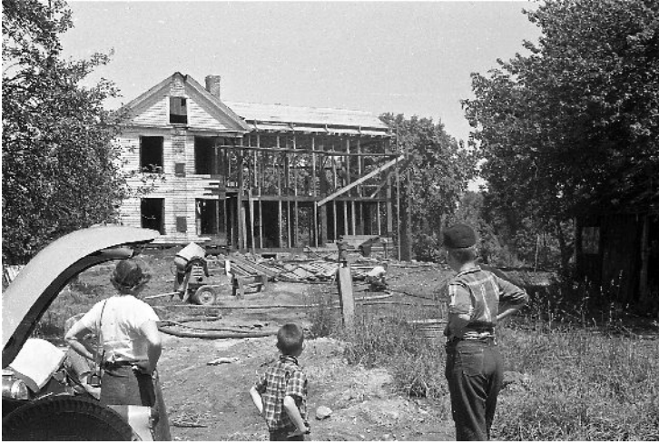
At left above and below: The Tyler farmhouse at 178 Lexington Street, during and after reconstruction in 1954. At right: 1954 photo of the Tyler farmhouse during reconstruction. (Photos by Peg Hunt, courtesy of Charles Hunt)
