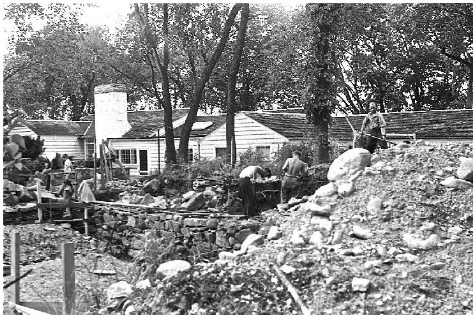
725 Boston Post Rd. The photograph shows the cellar hole of the former Flag Tavern, with the newly constructed Hunt house in the rear. Workman are in process of replacing the old tavern foundation with a swimming pool. Albert Hunt is the second person from the right, with his back turned. (Courtesy Charlie Hunt)
